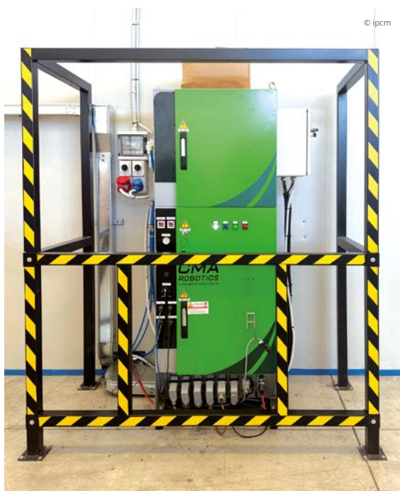
The robot's electrical panel.
