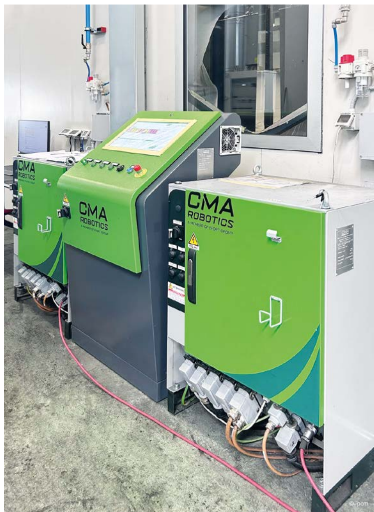
The control unit with the PLC managing the two articulated robots.
